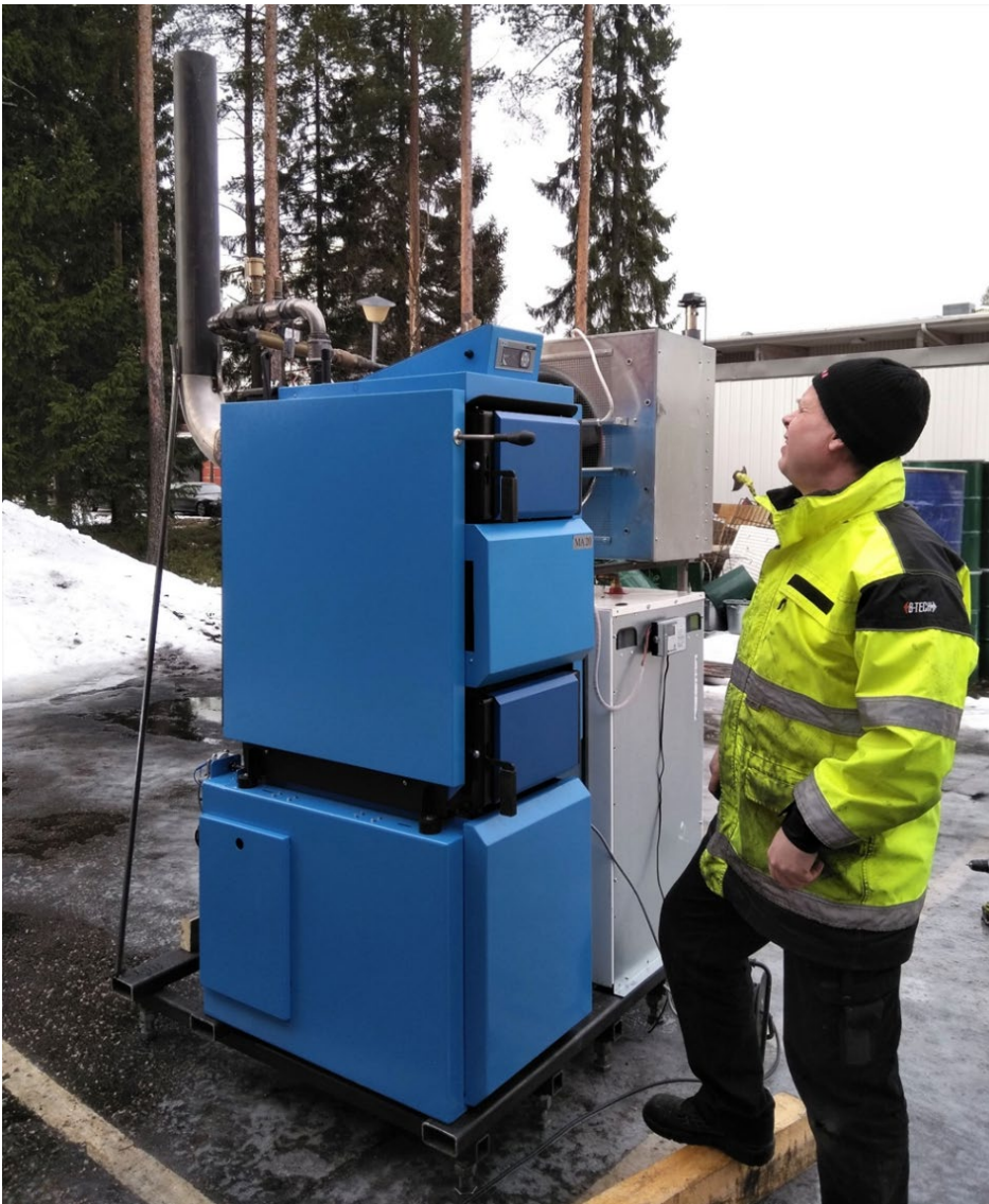
FIGURE 2. Trial operation of a wood log CHP unit (photo: Markku Kananen)
