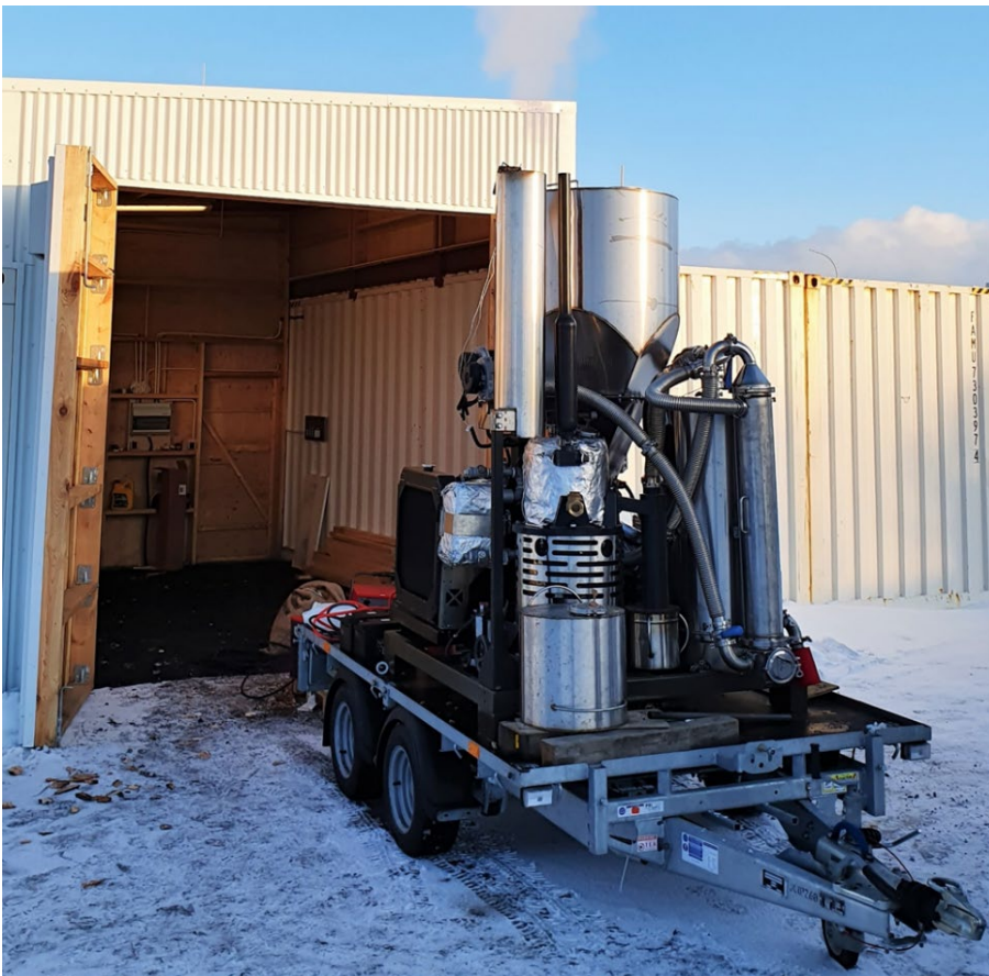
FIGURE 3. University of Iceland's CHP plant (photo: Rúnar Unnþórsson)
